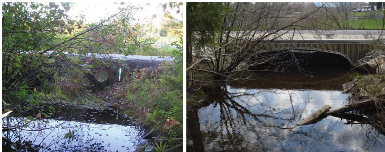
Figure 3-1. Totten Road crossing of Thayer Brook. Installation of a bottomless culvert: pre (L) and post (r) installation.
