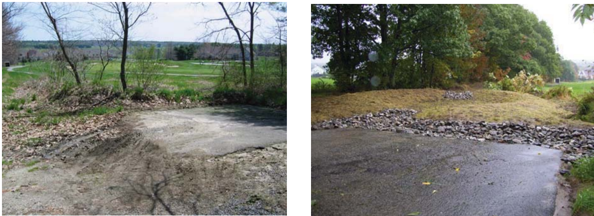
Figure 5-2. Falmouth Country Club equipment wash area BMP project: before (l), and after (r).
