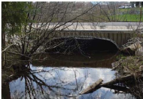
Totten Road crossing of Thayer Brook in Gray. Installation of a bottomless culvert pre- (above), and post- (below) installation.
