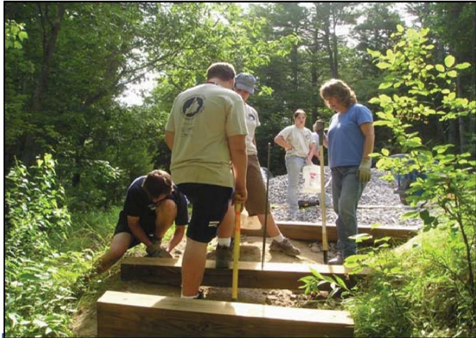
Figure 4-2. PRYCC crew members install infiltration steps on an eroding swimming hole access trail adjacent to a local road.
