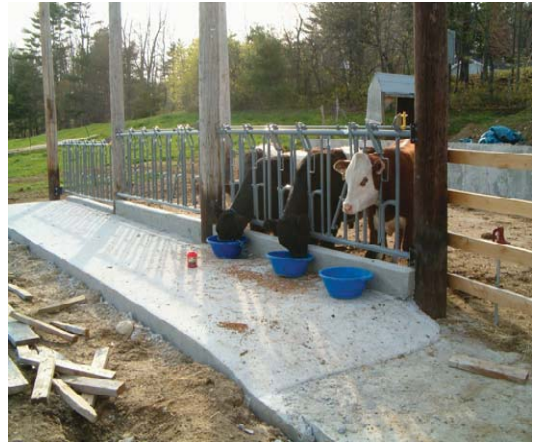
Figure 2-7. A concrete feeding and watering pad was installed at Breezy Knoll Farm to address erosion.
