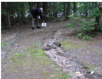
Runoff from the driveway and rooftops on this property combine to transport significant sediment into Parker Pond.
