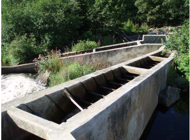
Photo 1-4. The Denil fish pass at the Bridge Street dam.
