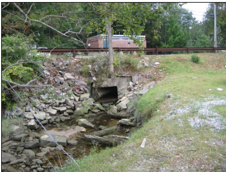
Photo 2-52. Perennial stream associated with Wetland 24, exiting north of Route 88 to the river. Stantec, September 20, 2007.
