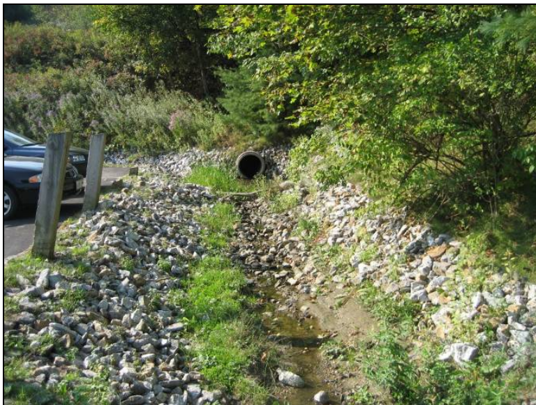
Photo 2-25. Drainage basin for Wetland 11, located on the north side of Route 88 in the Lower Falls Landing parking area. Stantec, September 20, 2007.
