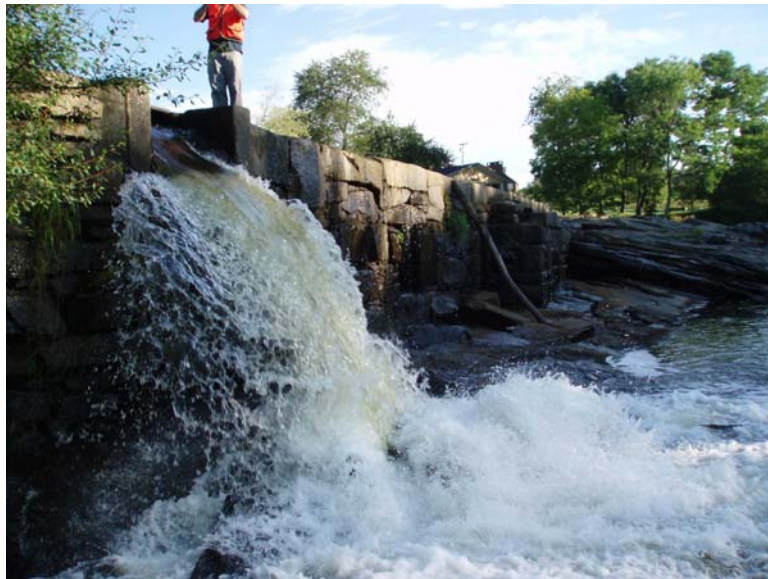
Photo 1-7. The East Elm Street dam, with leaks visible between stones.
