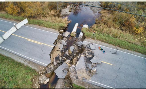
Culvert washout on Pushaw Rd in Glenburn, ME in October 2022 associated with a 25-year storm event. The washout resulted in a 5-mile detour and cost $111,000 to repair.
