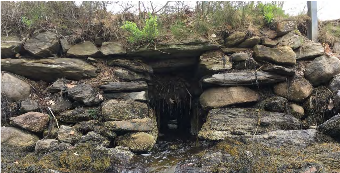
Primary Crossing of Small Point Road (outlet) - Dry Laid Stone Culvert w/ Timber Deck Beams
