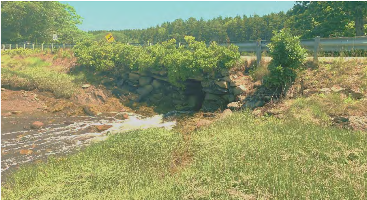
Primary Crossing of Small Point Road – Dry Laid Stone Culvert w/ approx. 2' Span
