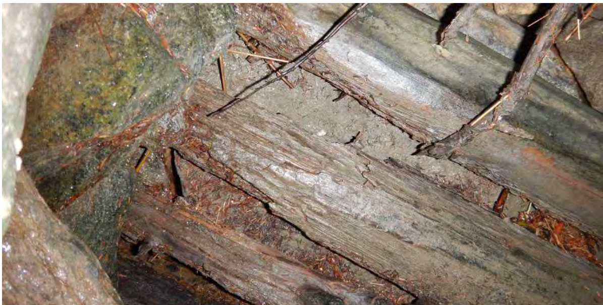
Primary Crossing of Small Point Road - Interior view of Deteriorated Timber Deck
