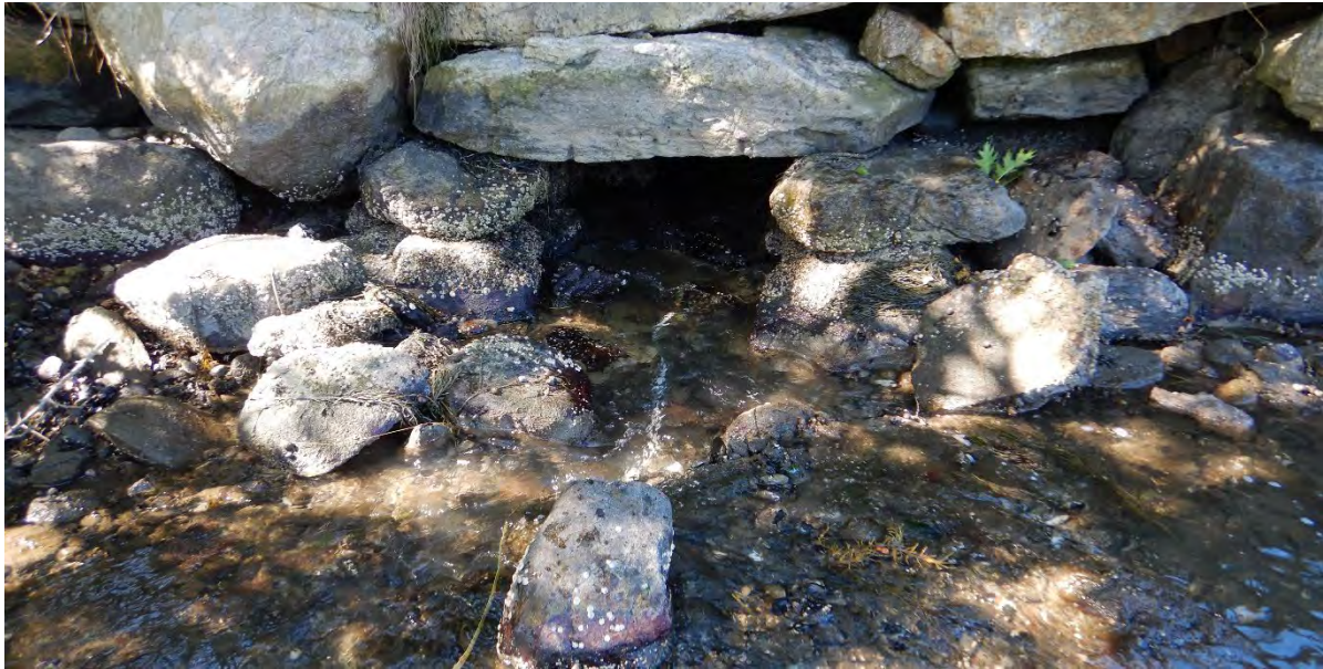
Primary Crossing of Small Point Road (inlet) - Dry Laid Stone Culvert w/ Timber Deck Beams
